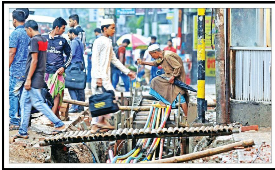
Poor safety measures during construction
