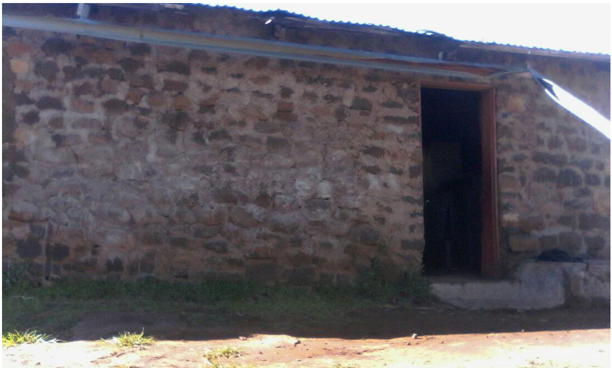
Figure 3 The pictures above show a building used for upper grades (4-7) in Ribaneng LECSA Primary school. The top one is the inside while the bottom one is the outside.
