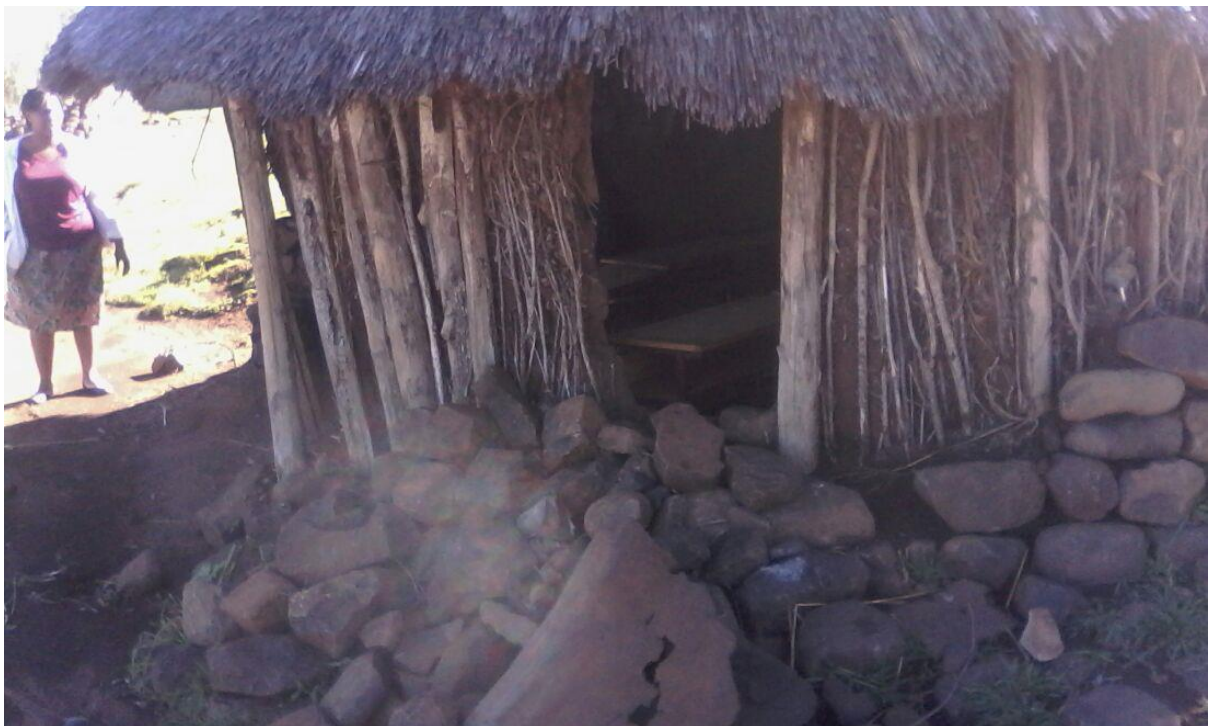
Figure 2 the picture shows the classroom mentioned in figure 1 above, from the outside.
