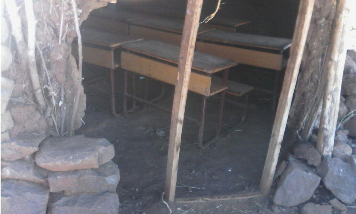
Figure 1 This is a building used as a classroom for the lower grades (1-3) this building falls apart every time there are heavy storms.
