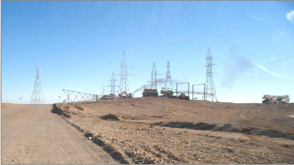
Figure 10: New power lines being installed near the Oyu Tolgoi mine license area.
